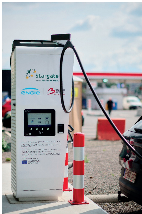
Figure 4 e-charging facilities promote more sustainable transport choices
